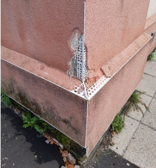
Figure 55 - Render delaminating on the Church
